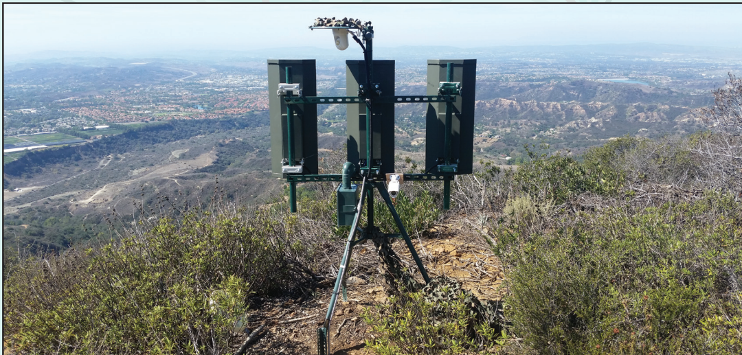
AE6XE Orange County California 3 node installation
